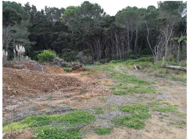
Early shared path works around the Museum area over the fascine drain
