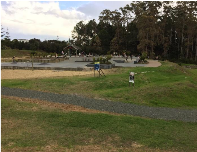
Existing MAZ area recontoured and paved draining to the low point on the Southwest
